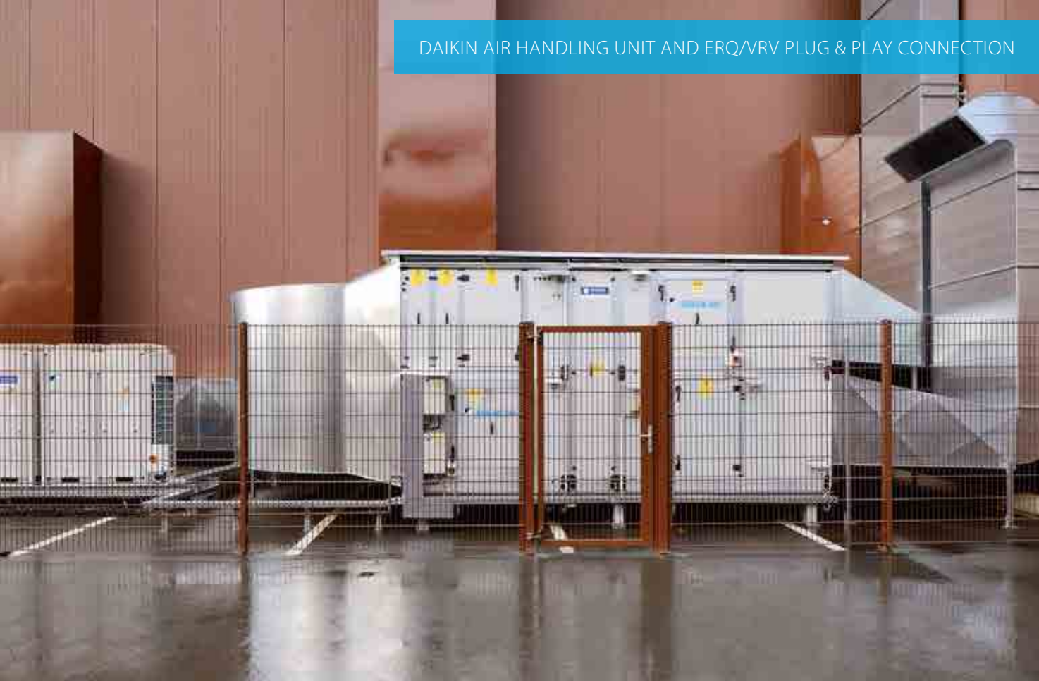
Ventilation & Air Handling
